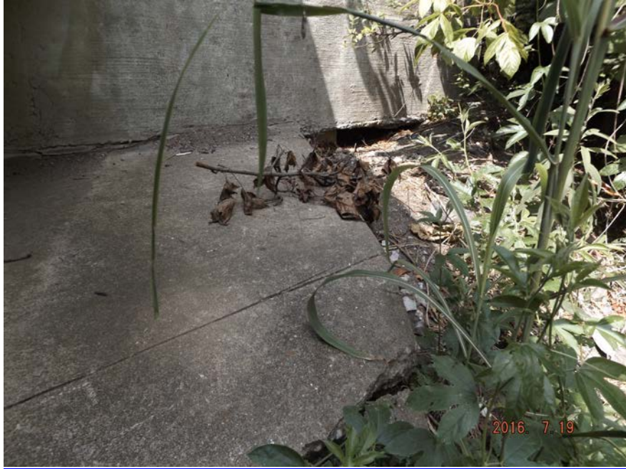
ABUTMENT 1 - LEFT - UNDERCUTTING
