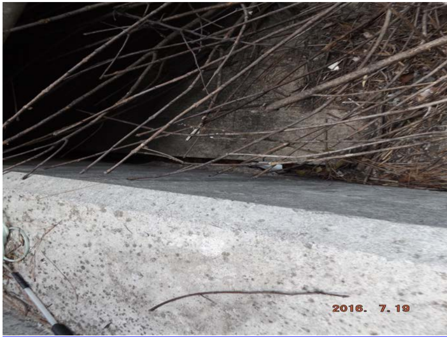
ABUTMENT 2 - LEFT - SEPARATION OF CONCRETE SLOPE
